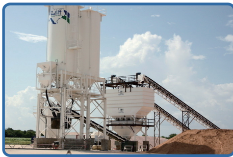
混凝土搅拌系统应用 Application in concrete mixing system
